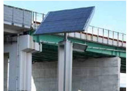
Solar LED Lighting
