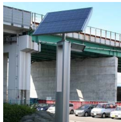
Solar LED Lighting
