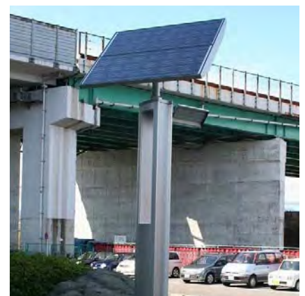
Solar LED Lighting
